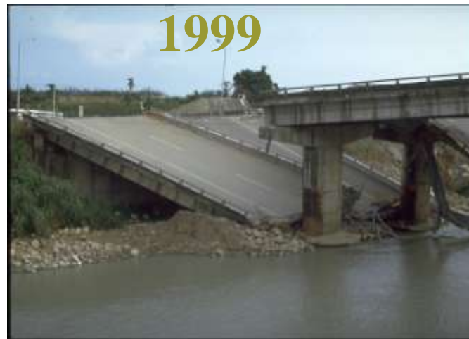
Bridge in Taiwan after 1999 Chi-Chi earthquake
