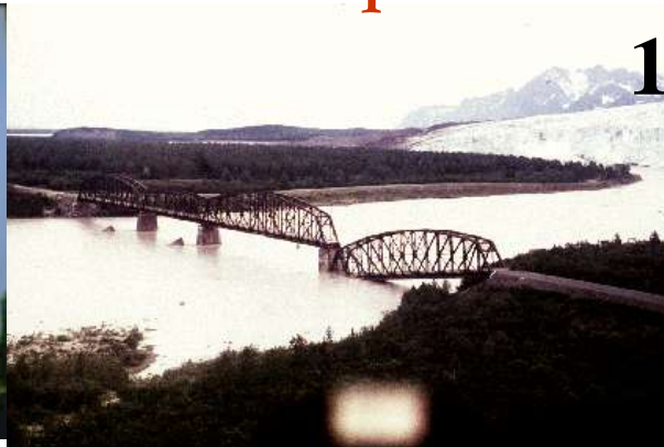
Million Dollar Bridge after 1964 Alaska earthquake
